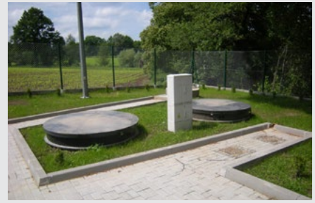
▶ Remote settlement and buffer tanks to suit a site with restricted space.
