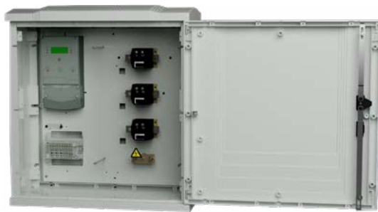
Example: electrical indirect metering
